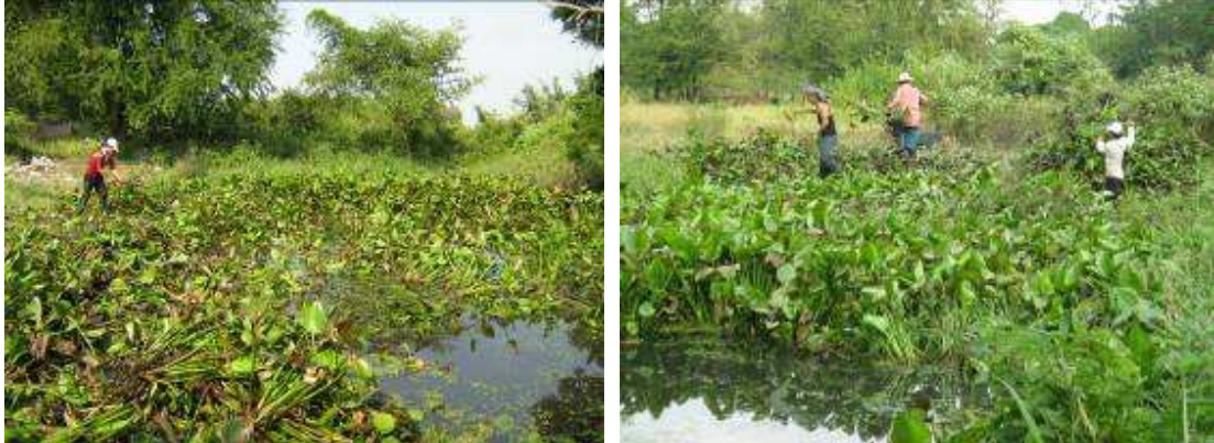
2 big ponds have to be emptied and prepared for the future building site
